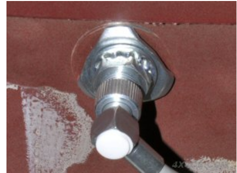
A quick way to get a metal-to-metal connection is to rotate the 3 pronged washer while applying pressure - the points will cut through the paint, although they will also move outwards slightly as they are compressed when tightened up so make sure they still touch bare metal!
