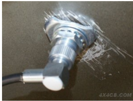
Here you can see where the paint on the underside of the roof has been scraped away to get a good metal-to-metal earth connection
